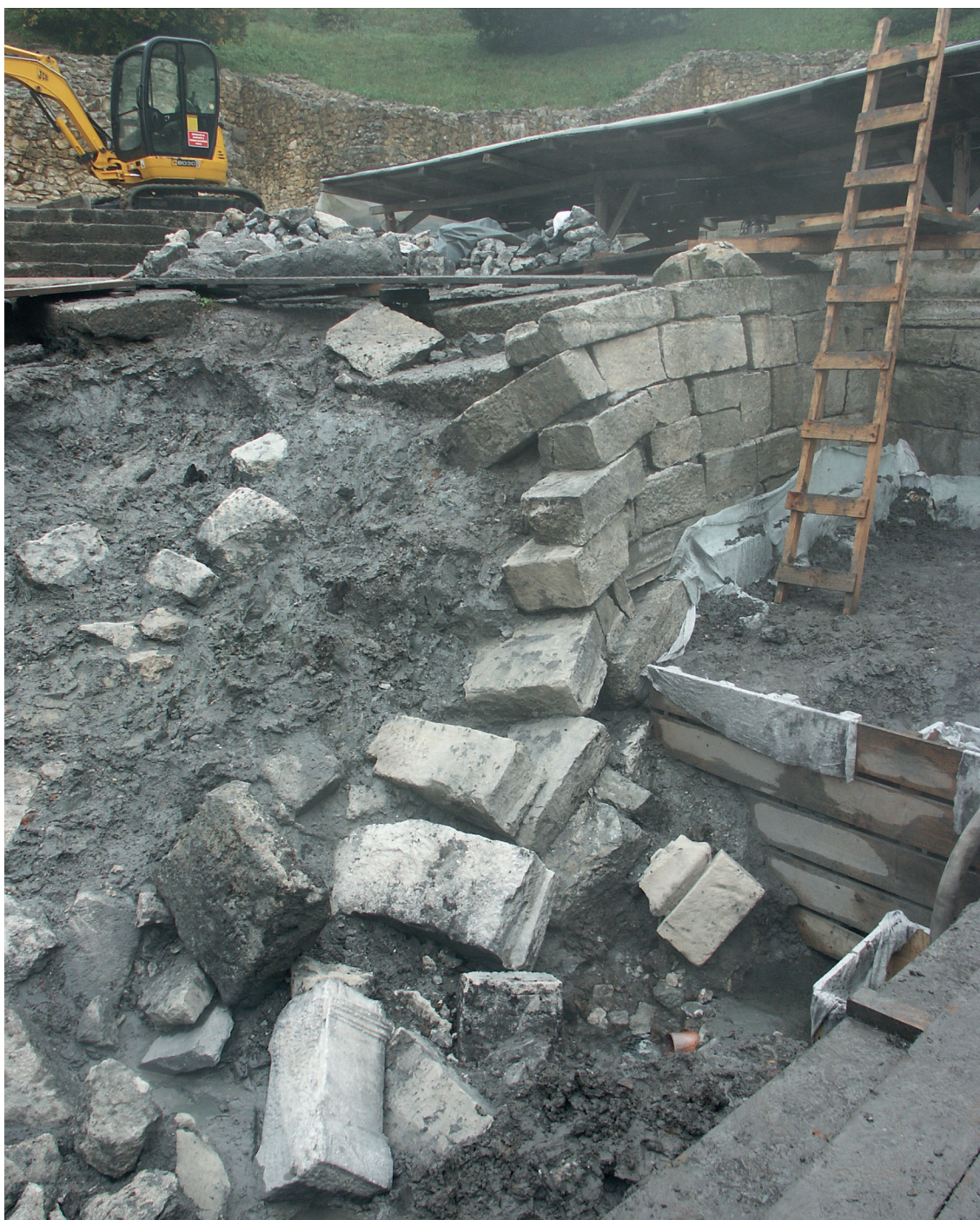
Slika / Figure 8: Pogled na urušeni sjeverni zid izvorišnog bazena, tijekom istraživanja 2011. god. (snimila D. Nemeth-Ehrlich). / A collapsed northern wall of the spring reservoir during the 2011 excavations (photo by D. Nemeth-Ehrlich).
